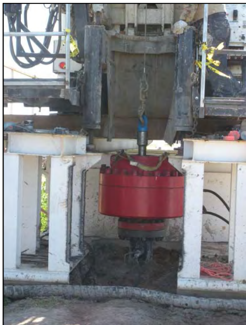
Figure C2. Photograph of blowout prevention (BOP) for annular space at base of drilling rig platform at MW02.
