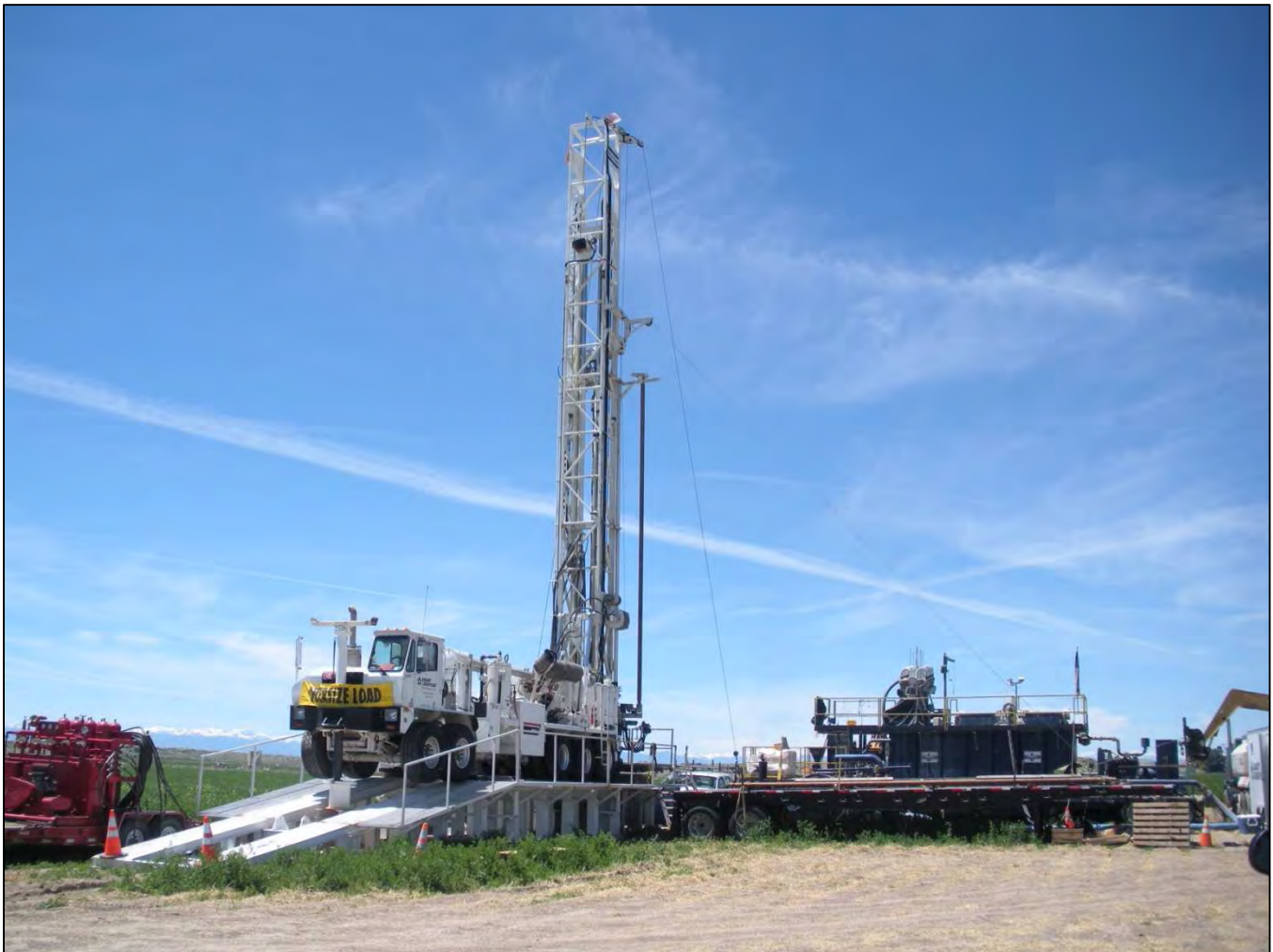
Figure C1. Photograph of drilling rig on platform with shakers for mud recirculation at MW02.
