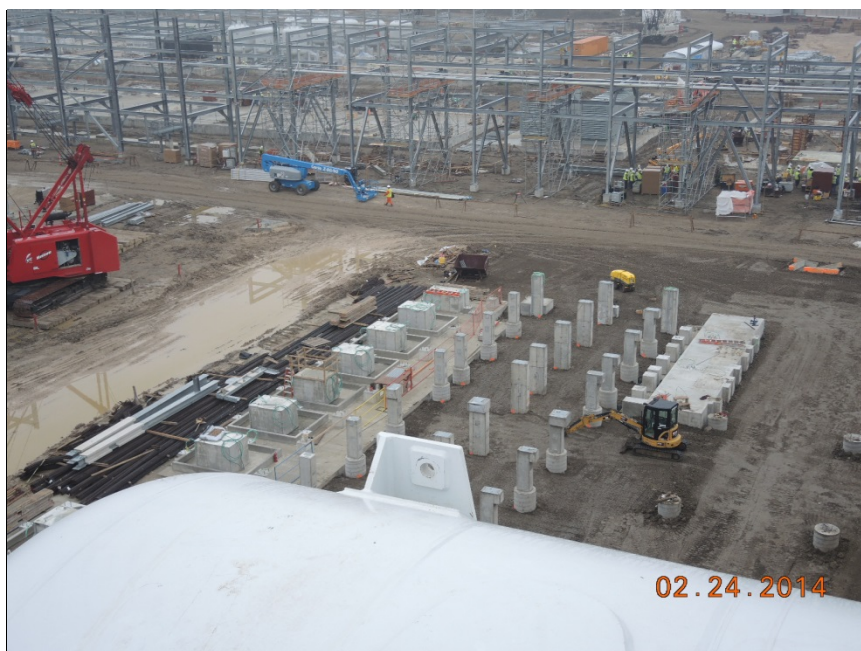
Train 1 131N02 (propane substation) (24-Feb-2014)
