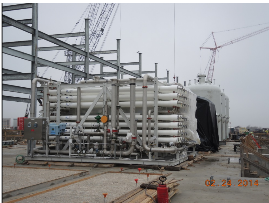
OSBL 135F01 (water treatment area) (24-Feb-2014)
