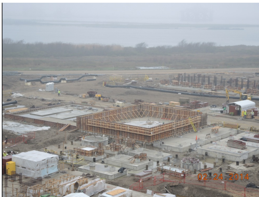
Train 2 132B01 (amine storage area and thermal oxidizer) (24-Feb-2014)
