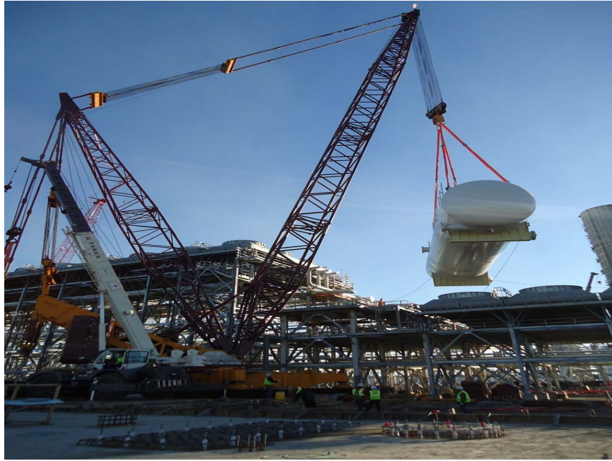
Train 1 131N01 (set accumulator) (24-Feb-2014)
