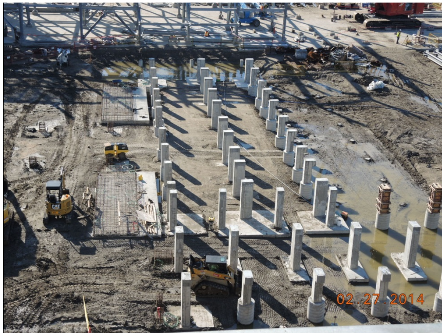
Train 2 132A02 (compressor substation) (27-Feb-2014)
