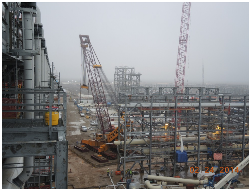
Train 1 131K01 (dehydration mercury removal) (24-Feb-2014)
