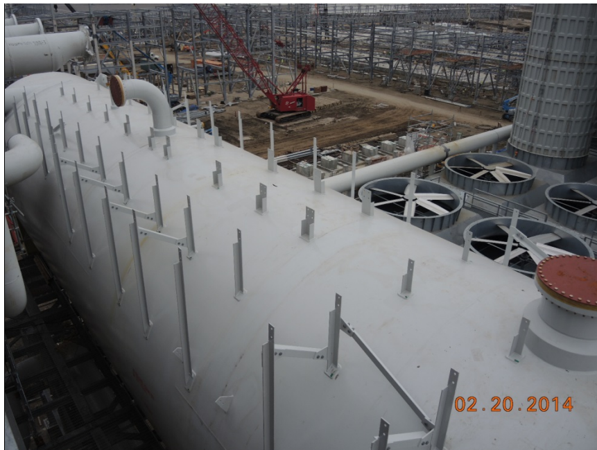
Train 1 131N01 (propane rack accumulator set) (20-Feb-2014)
