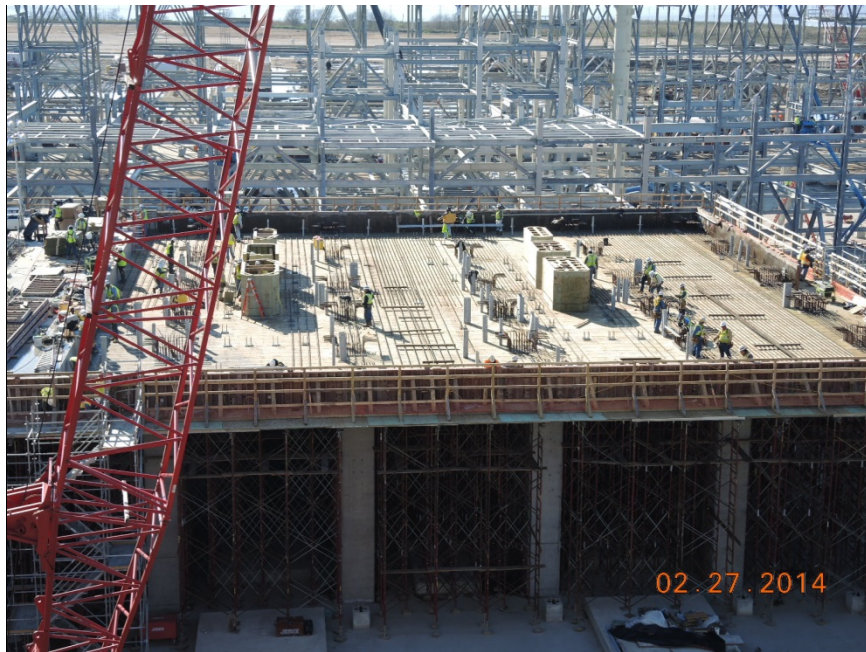
Train 2 132A01 (compressor methane tabletop) (27-Feb-2014)
