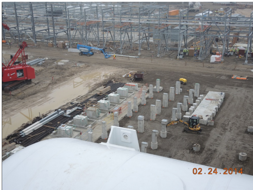
Train 1 131N02 (propane substation) (24-Feb-2014)
