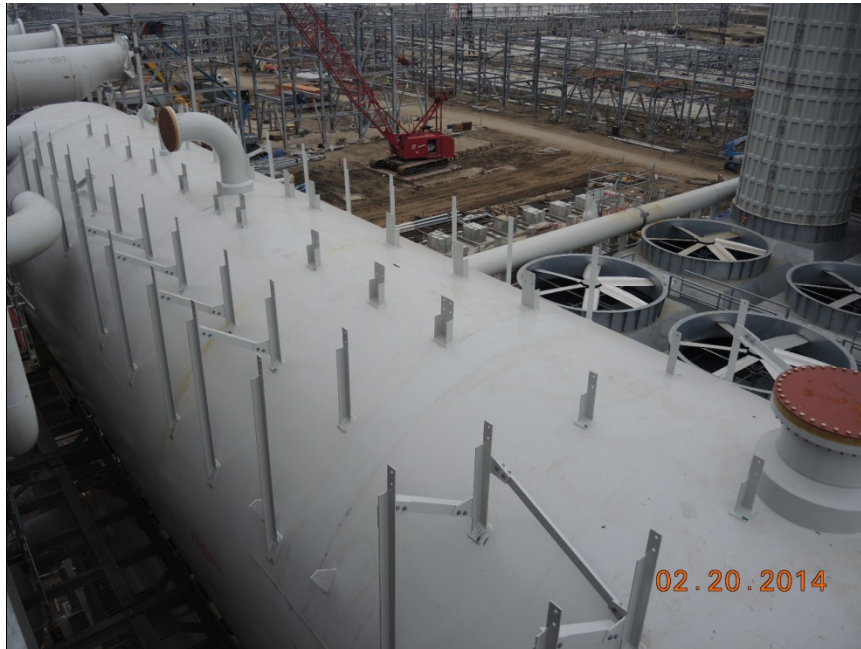
Train 1 131N01 (propane rack accumulator set) (20-Feb-2014)
