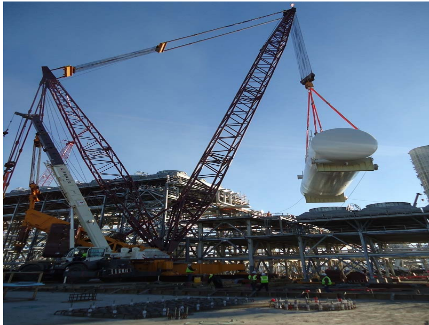
Train 1 131N01 (set accumulator) (24-Feb-2014)
