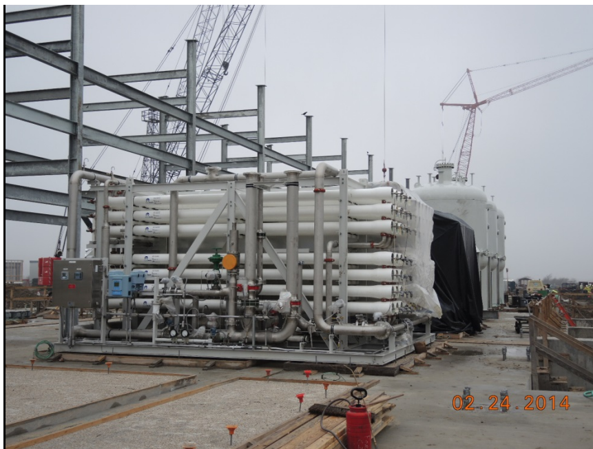
OSBL 135F01 (water treatment area) (24-Feb-2014)
