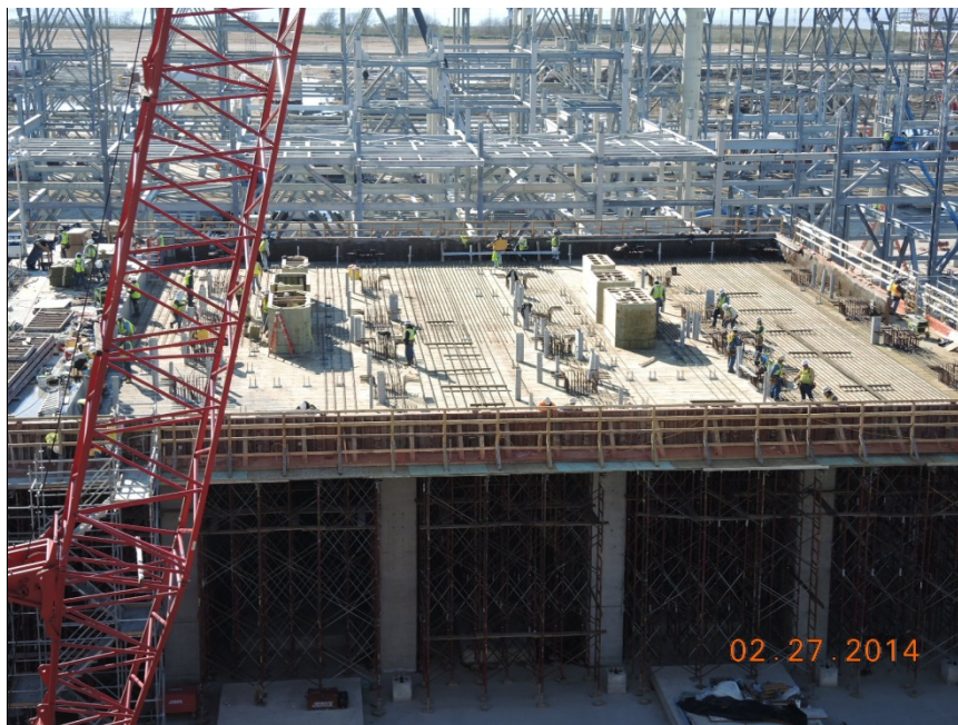
Train 2 132A01 (compressor methane tabletop) (27-Feb-2014)
