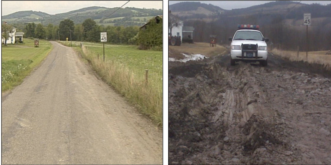
Figure 5: Before and after photos of SR 3020 in Bradford County, PA, due to heavy truck traffic during the dynamic spring thaw. Source: PA DOT.
