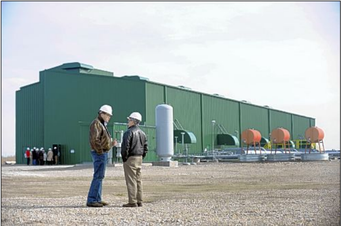
Gas Compressor Station
