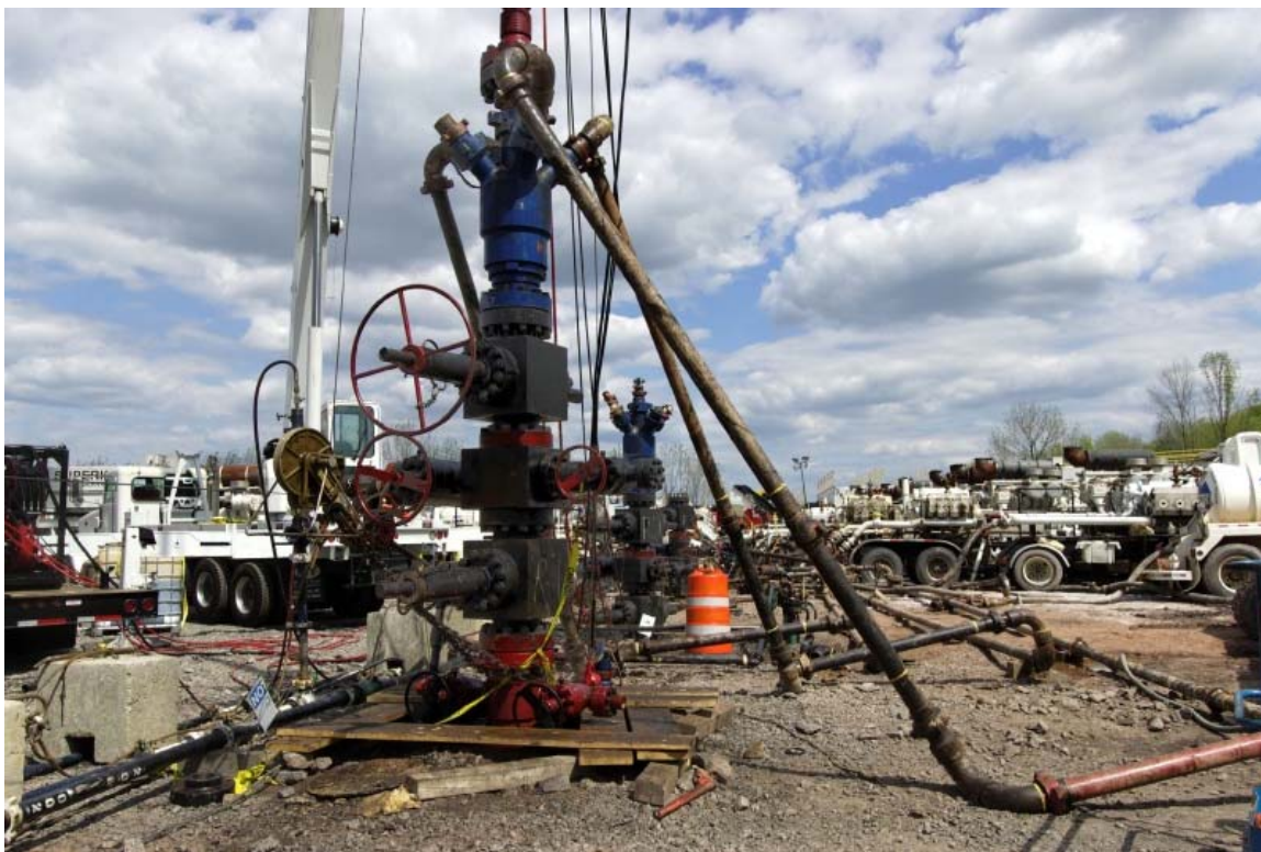
Photo 5.24 - Three Fortuna Energy wells being prepared for hydraulic fracturing, with 10,000 psi well head and goat head attached to lines. Troy PA. Source: New York State Department of Environmental Conservation 2009
