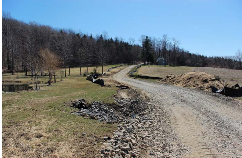
Photo 5.2 Nornew, Smyrna Hillbillies #2H, access road, Smyrna, Madison County NY. Photo taken during drilling phase of improved existing private dirt road (approximately 0.8 miles long). Not visible in photo is an additional 0.6 mile of new access road construction. Operator added ditches, drainage, gravel & silt fence to existing dirt road. The traveled part of the road surface in the picture is 12.5' wide; width including drainage ditches is approximately 27 feet. Portion of the road crossing a protected stream is approximately 20 feet wide. Source: NYS DEC 2008.
