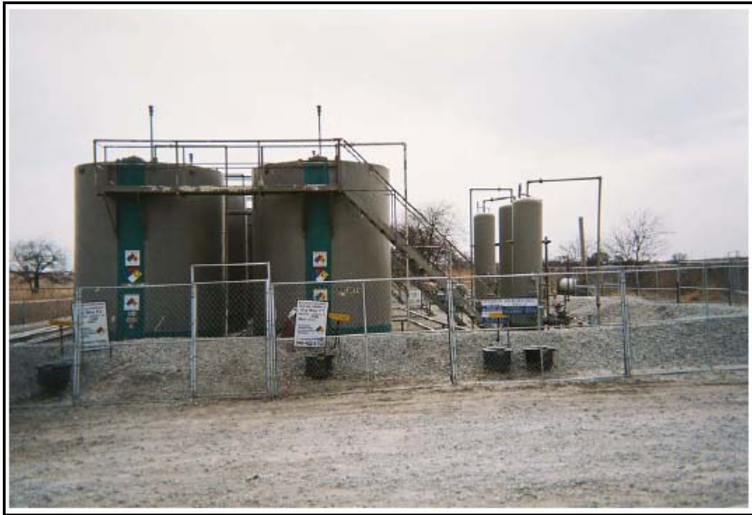
Figure 5. Example Storage Tank Battery (left), Separators (right), and Piping. (14)
