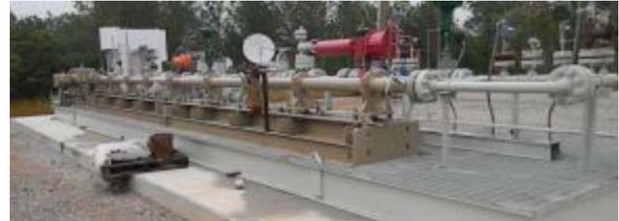
CO 2 Injection Pump (Denbury)
