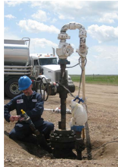
Photo from 2009 EERC CO 2 injection test into a conventional oil well in the Northwest McGregor field, North Dakota.
