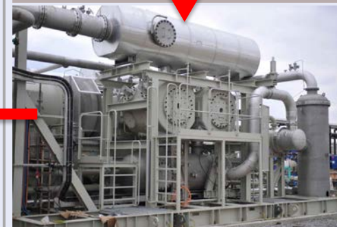
Wet CO 2 compressor
