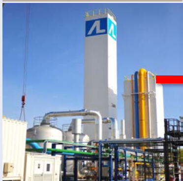
Air separation unit
