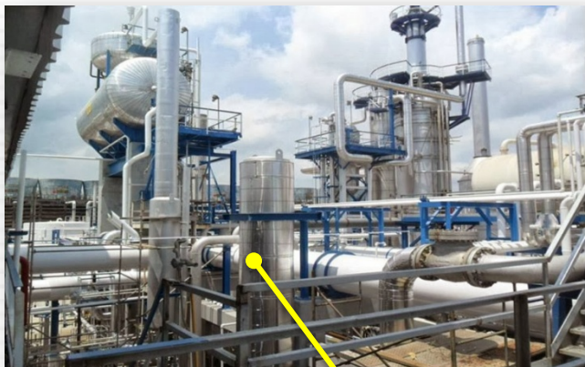
PEMEX Ammonia Plant Cosoleacaque
