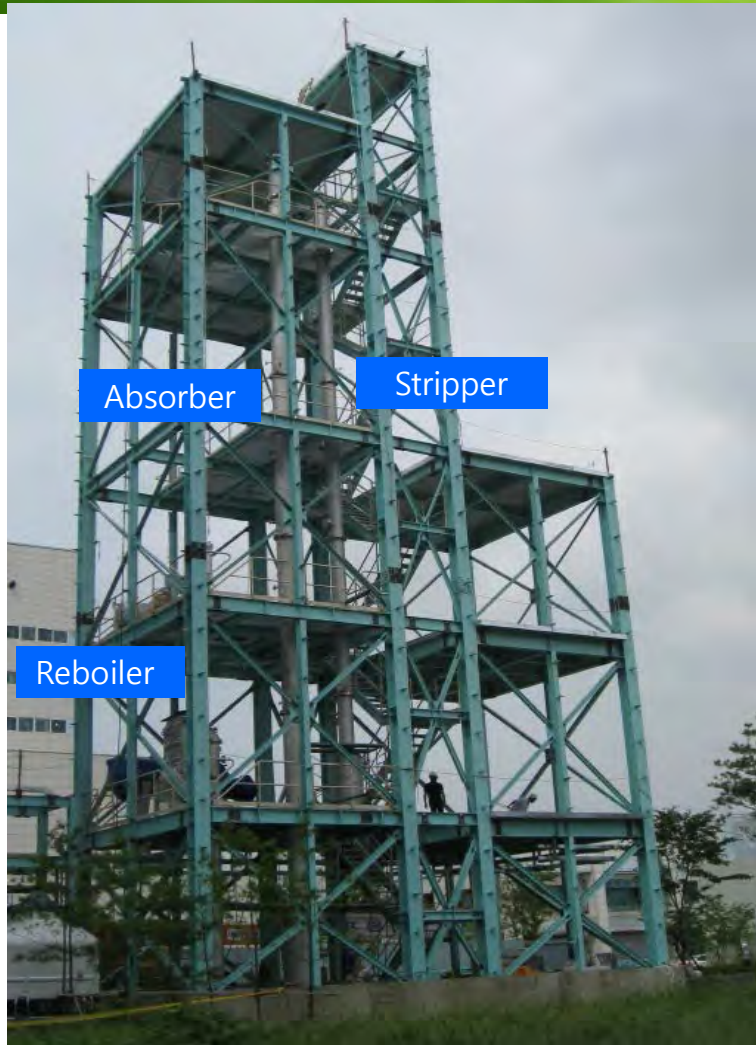
0.1MW Test-bed at Boryeong coal-fired power plant
