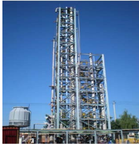
CCM verification Plant for coal and natural gas tons 1000 CO 2 /year
