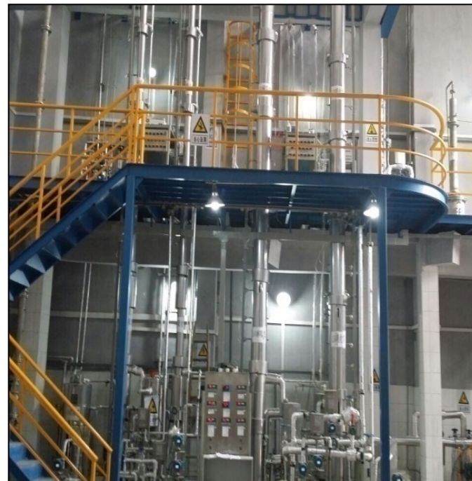
Pilot-plant of CO 2 removal and separation in Yanchang Petroleum Group
