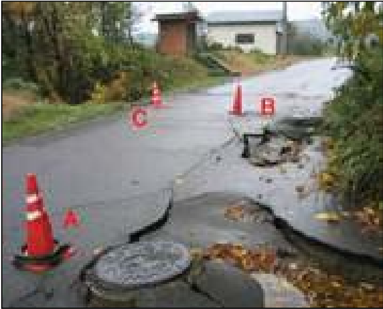
Access Road to the Site Damaged
