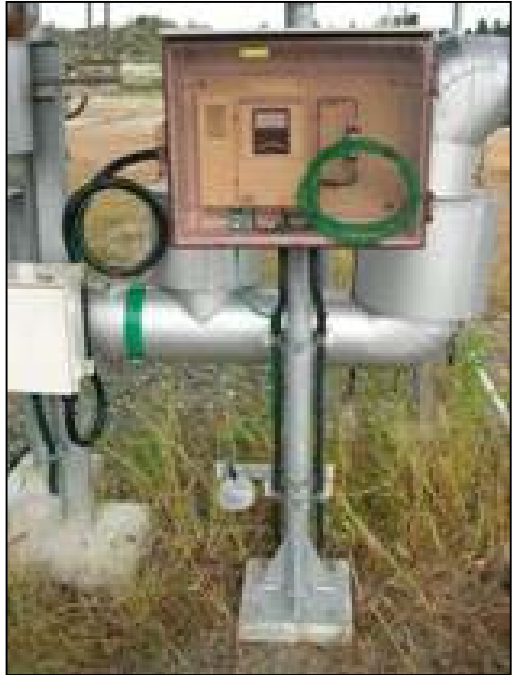
Onsite CO 2 Detector Detected No Leakage
