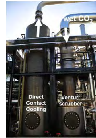
Flue gas cooling tower
