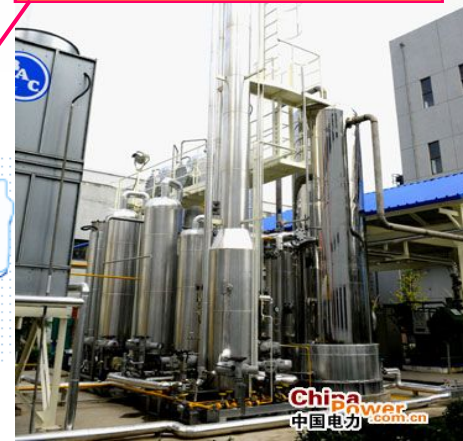
Huaneng Shidongkou Power Station 10×10 4 t/a (Operation)
