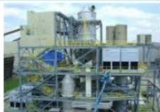
AEP Mountaineer USA - 58 MWth Chilled Ammonia - Coal
