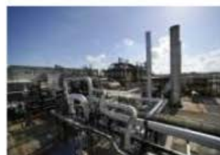
Total Lacq France - 30 MWth Oxy - Gas
