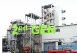
DOE/Alstom Windsor US - 3 MWth Chemical looping - Coal
