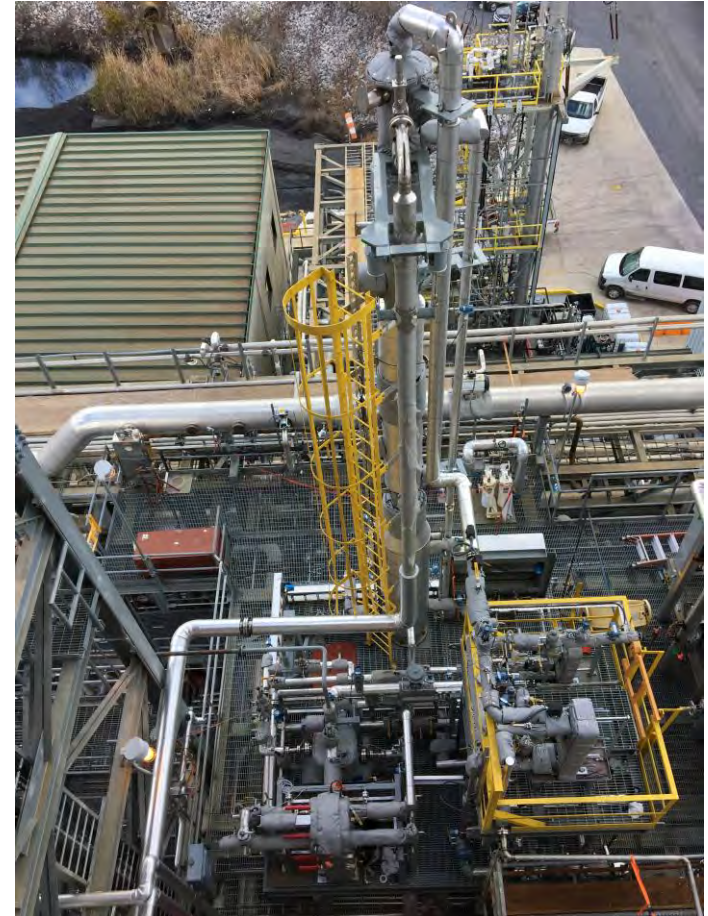
AFS Skid installed at NCCC Photograph courtesy of UT, NCCC
