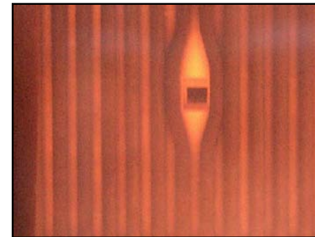
Existing measurement port
