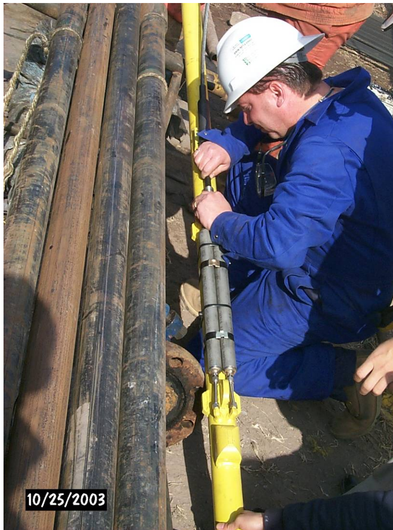
Figure 5: Pressure Gauge Installation
