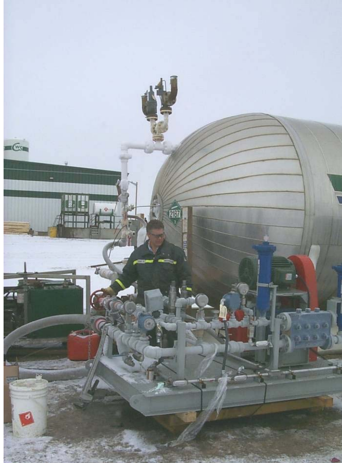
Figure 6: Testing the CO 2 Pump at Calfrac Facility at Red Deer, Alberta
