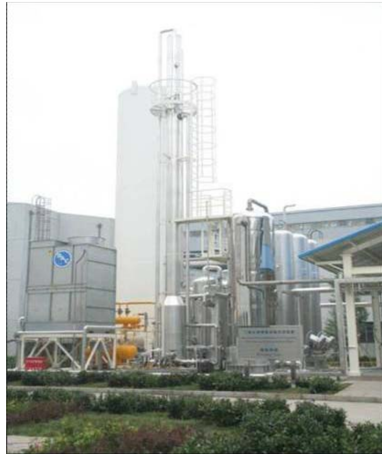
Huaneng Beijing Gaobeidian Thermal Power Plant, start operation in 2008, CO 2 used in food industry
