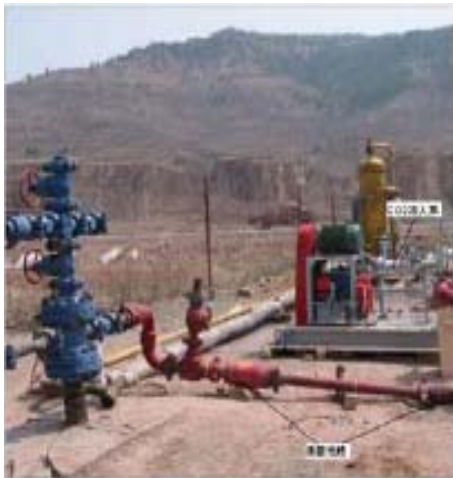
CUCBM CO 2 -ECBM Well Site
