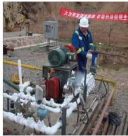
CUCBM CO 2 -ECBM Well Site
