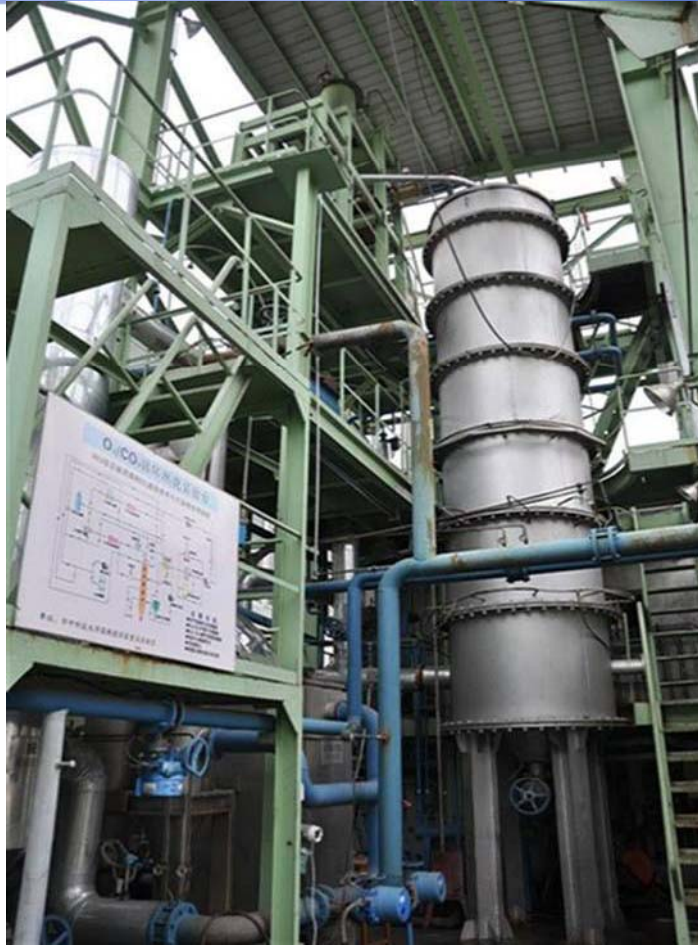
Existing 400kWt Oxy-fuel recycle combustion facility
