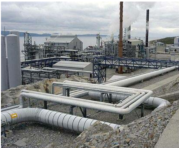
Power plant at Tjeldbergodden
