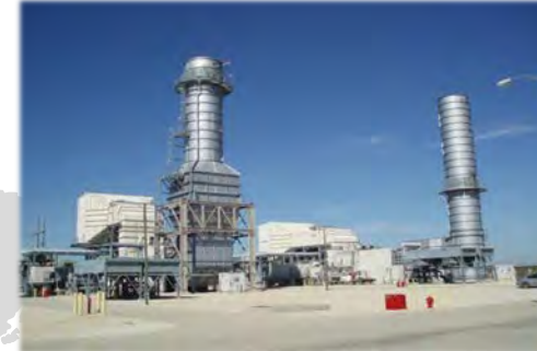
Elwood Energy Gas Power Plant (United States)
