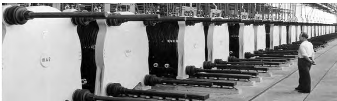
Figure A.8.2: Electrolyser production hall, Norsk Hydro Glomfjord, producing 30 000 Nm 3 /hr (NEL Hydrogen)
