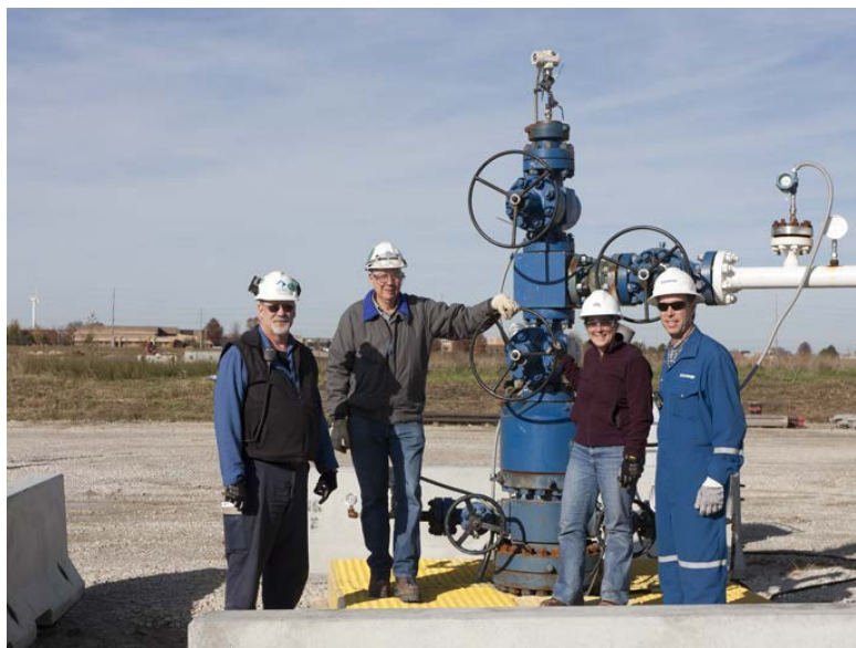
Figure 2-8: Injection Well for the Illinois Basin - Decatur Project
