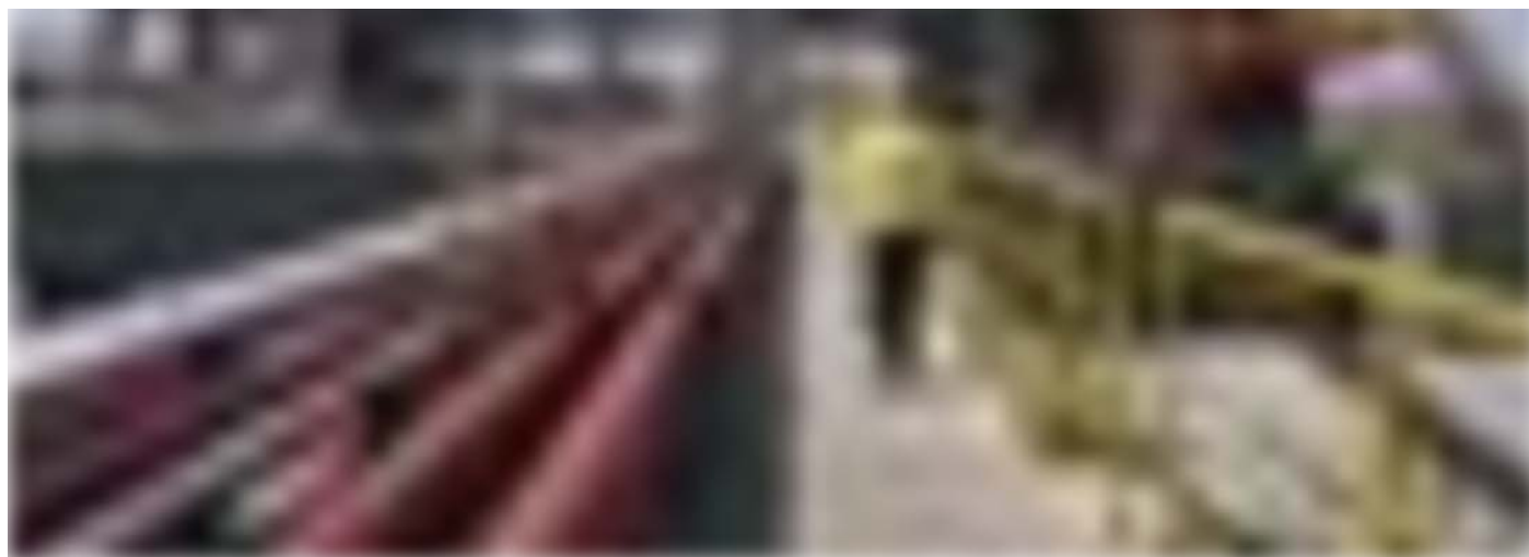
A worker walks past pipework at a LNG transfer pier facility Photographer: Qilai Shen/Bloomberg
